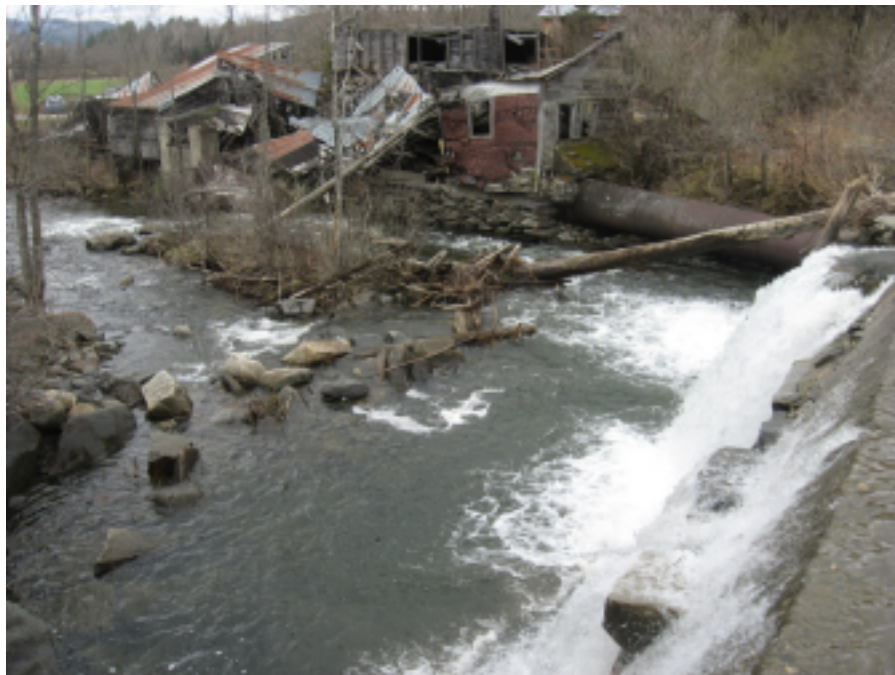
Figure 3: Deteriorated Remains of the Clark Saw Mill (Looking Downstream from the Dam) (Photo Taken by B. Cote, 5/5/2016)
