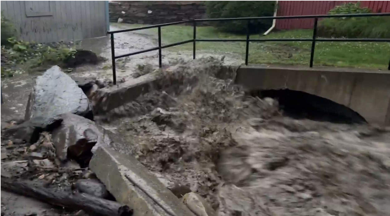
Figure 21: Flood waters overtopping culverts
