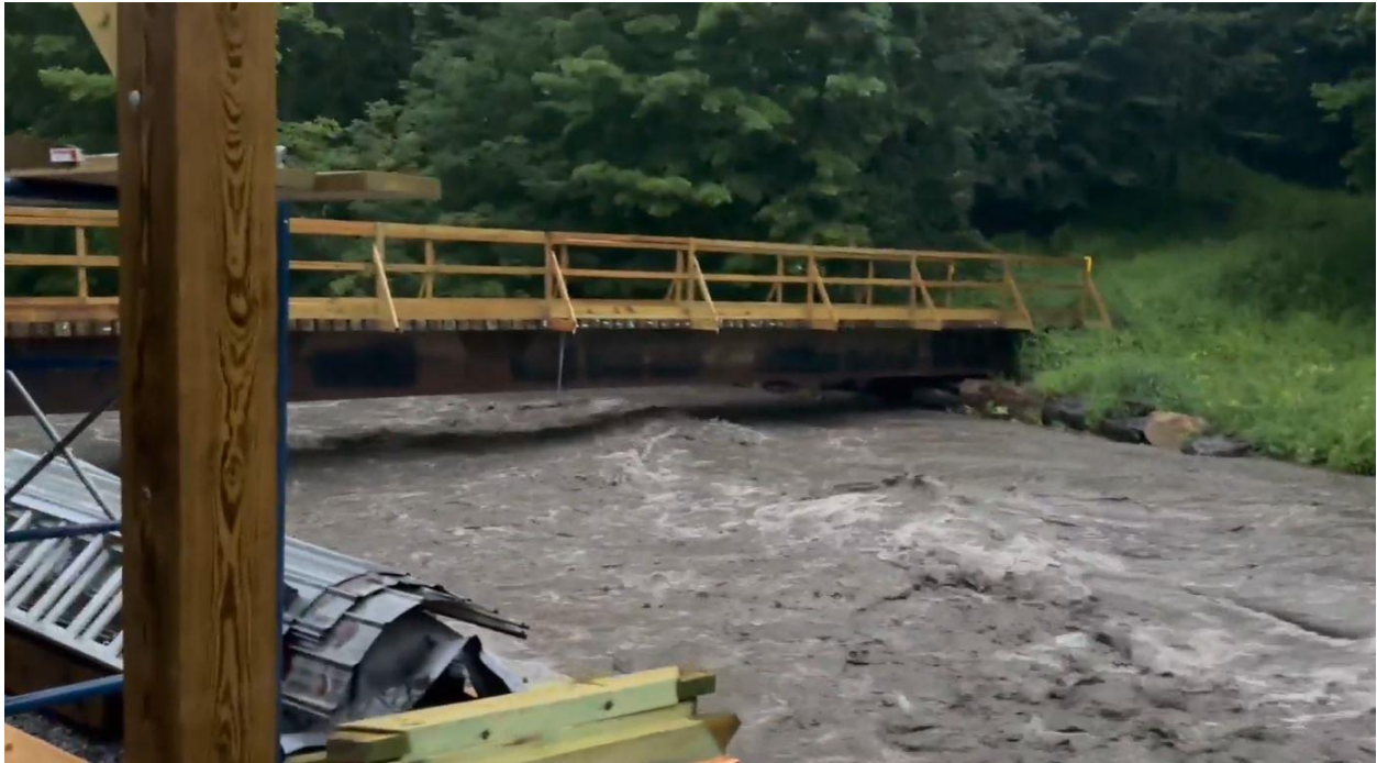
Figure 23: Flood waters passing under the VAST bridge
