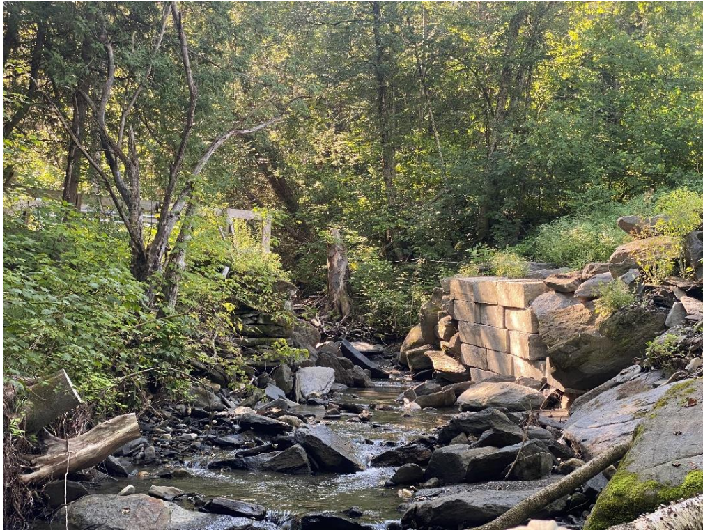
Figure 13: Constriction at the Damaged VAST Bridge
