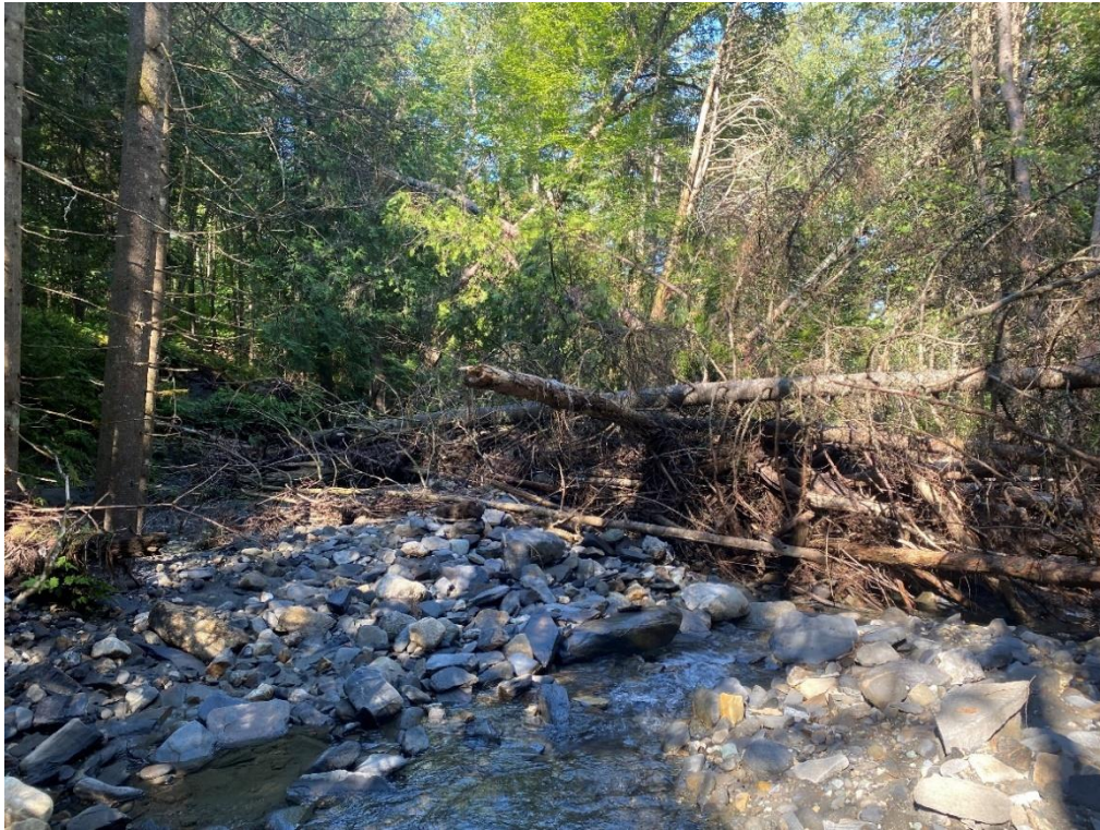
Figure 27: Large wood jam and sediment deposition upstream of the abutments
