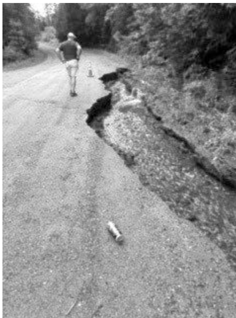
West Shore Road damage, 2024, picture taken by Emily Sable and Joshua Pollack
