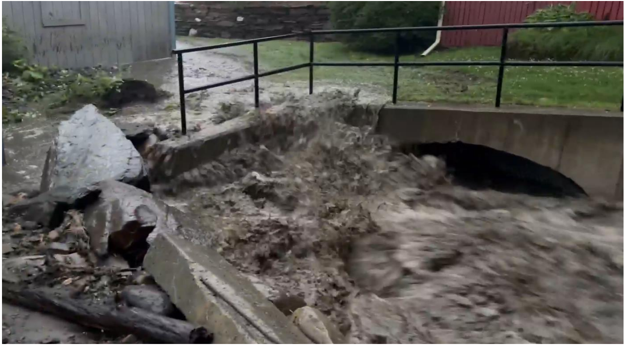
Figure 21: Flood waters overtopping culverts
